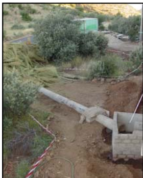
Damage to vegetation can be reduced by defining the impact area with hazard tape. The area outside the tape must be no-go for the builders. © P.Tarr
